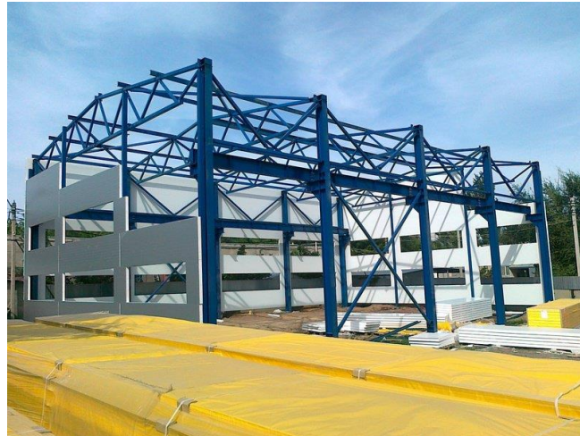
Pic. 2. Wall frame and roofing metal structures are sewn up with sandwich panels
