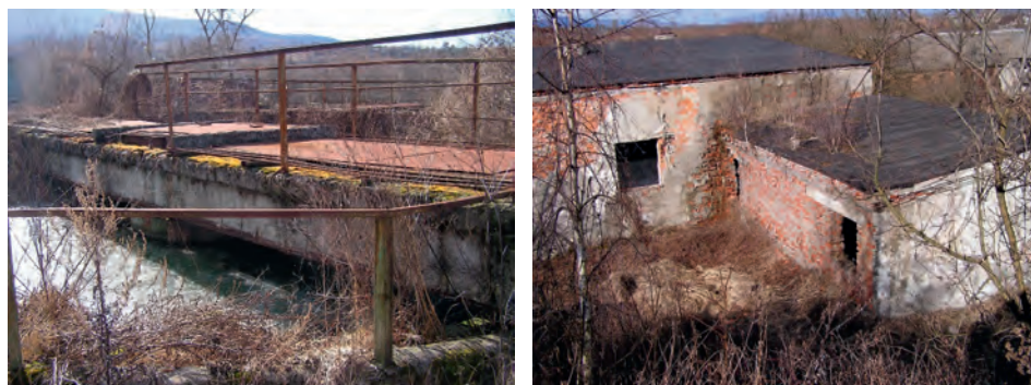
Fig. 1.2.13. Sewage Treatment Facilities in Tyachiv
