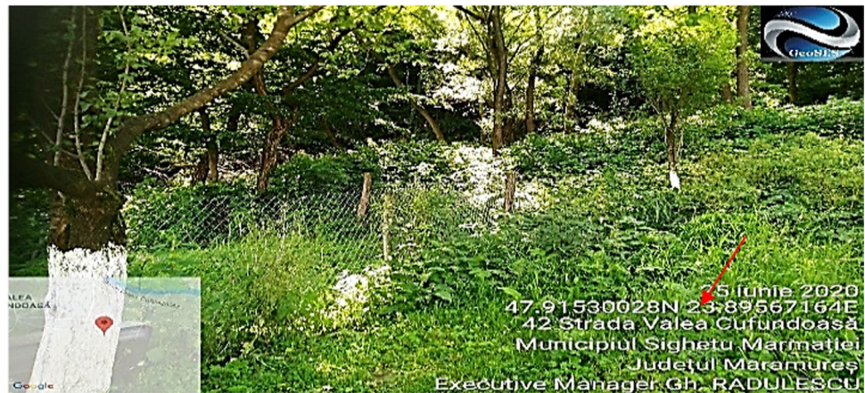
Fig. 9 Landslide located on Valea Cufundoasă Street, Sighetu Marmatiei Municipality (Source: GeoSES Project (Project GeoSES 2021))
