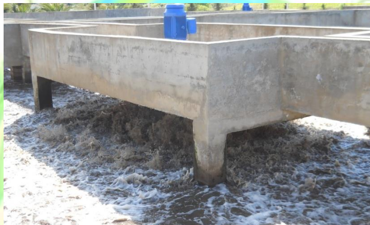
Figure 3: Biological Treatment, aeration basin
